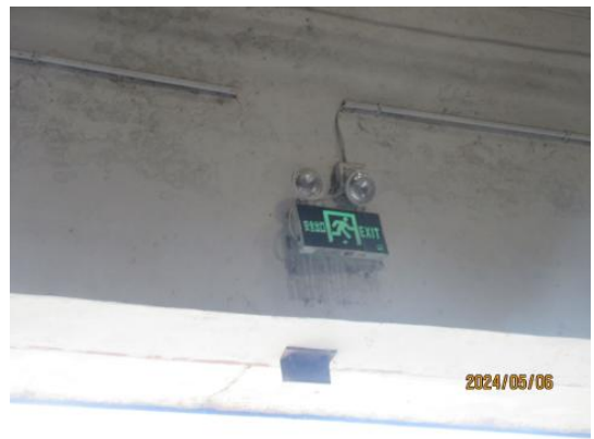
exit sign and emergency light.JPG
