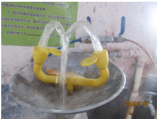
eye wash facility.JPG
